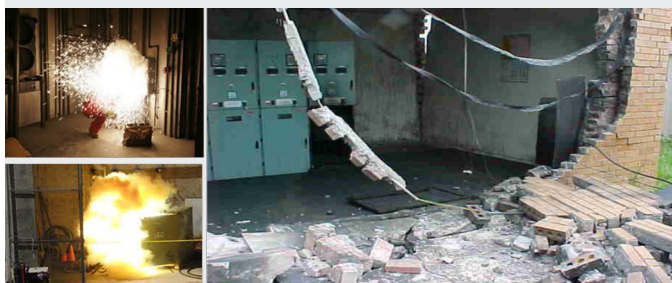
The likelihood of a shock exposure and arcing fault and arc flash increase when equipment is designed, installed, operated, or maintained improperly
